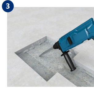
3 Use a hammer drill or other suitable tool to mill the surface inside the cut lines to a depth of 1.5 inches.
